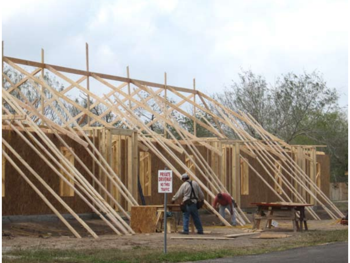
Multi-family construction continues in the Valley but single family construction is lagging behind. (VBR)
