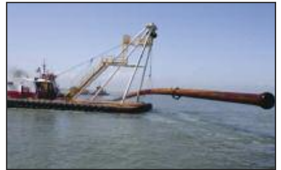
The barge raises the 700 foot section of 30 inch diameter floating pipe to bring it over the jetty at South Padre Island (courtesy)
