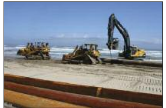
The floating pipe is pulled ashore with multiple cranes and then pushed by bulldozers. (courtesy)
