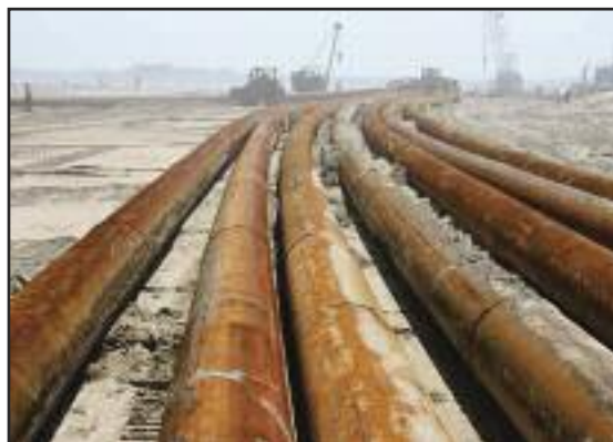
The pipe is stockpiled on the beach near the jetty, note how the 30 inch pipe bends. (courtesy)
